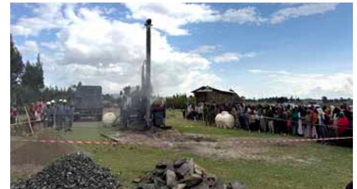
A drill crew and village watch as a Water for Good drill makes its final push towards hitting water — which happened just seconds later.
